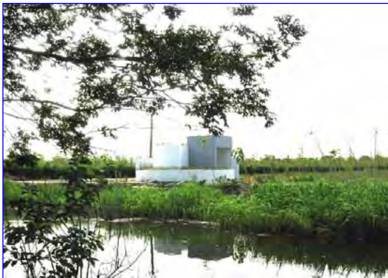
Figure 2. Demonstration Device of Tower Microbial-earthworm Ecofilter System (Tower Microbial-earthworm Ecofilter)
