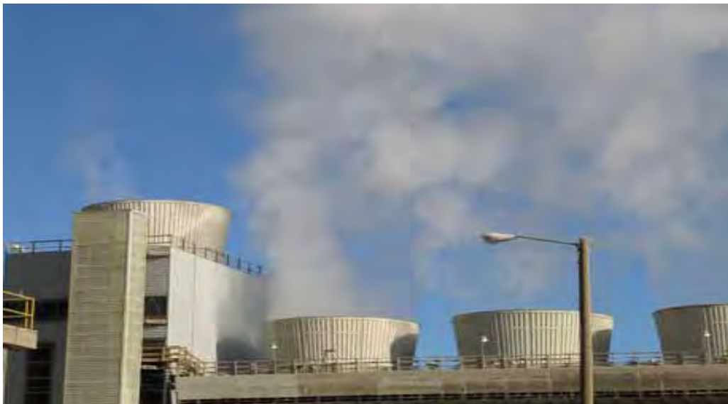
Figure 2. Photograph of the Air2Air® in operation at San Juan Generating Station. The Air2Air® is the taller stack on the left with a smaller plume.
